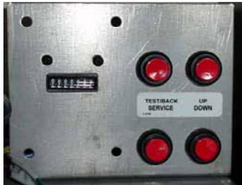
Figure 5. Operator Button Panel
